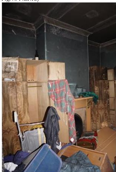
Fig.17 The front room has extensive fire damage
